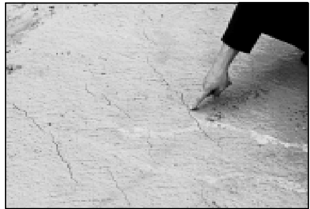
Plastic Shrinkage Cracks
